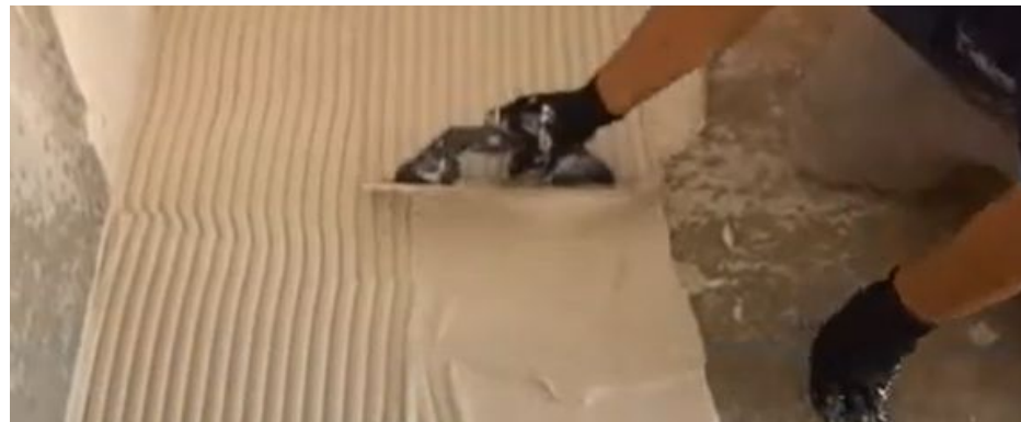
Image 26: Opening of mortar grooves on the laying area with the toothed side of the trowel.
