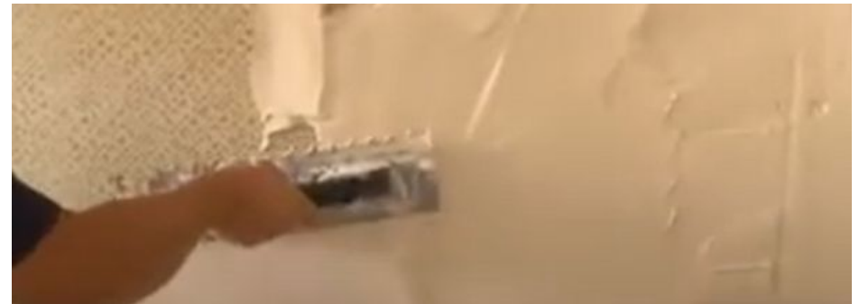
Image 27: Application of mortar to the ceramic coating with the smooth side of the trowel.
