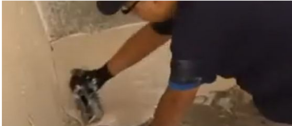
Image 25: Apply mortar to the laying area with the smooth side of the trowel.
