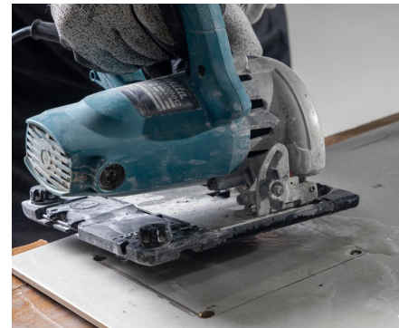
Image 82: Finish opening the four holes with the marble saw.
