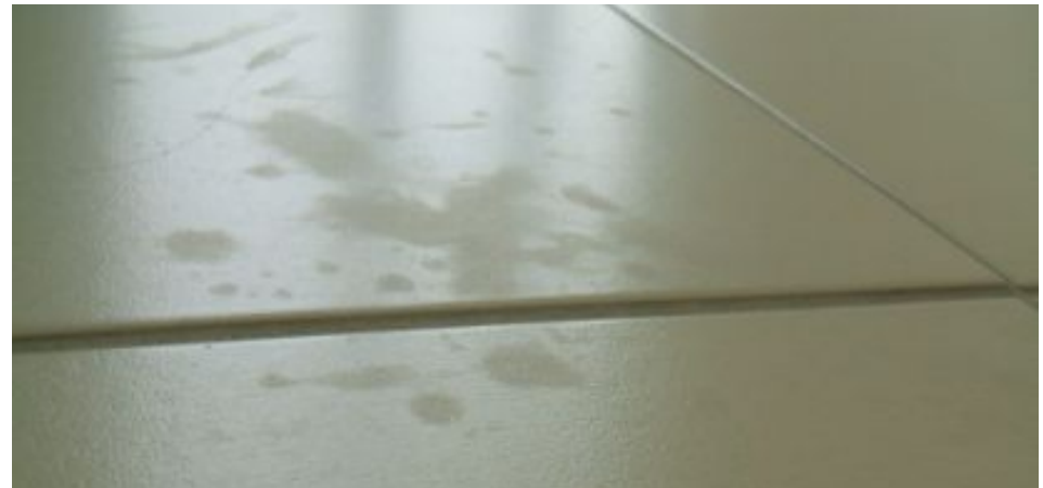
Image 103: Chemical damage caused by the dripping of a non-recommended product.
