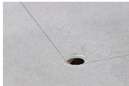
Image 86: Finish opening the four holes with the marble saw.
