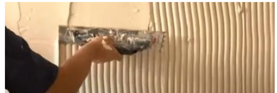
Image 28: Opening of mortar grooves in the ceramic coating with the toothed side of the trowel.
